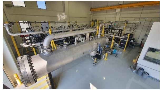
Figure 3: Picture of 4-inch flowloop facility
