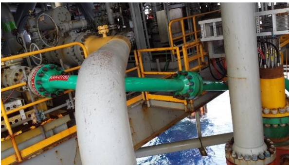
Figure 4. Old Production Piping Connecting to BV.
